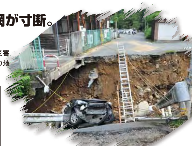
橋梁崩壊(田籠・日森園橋)
